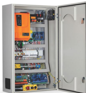
Integrated Control Panel
